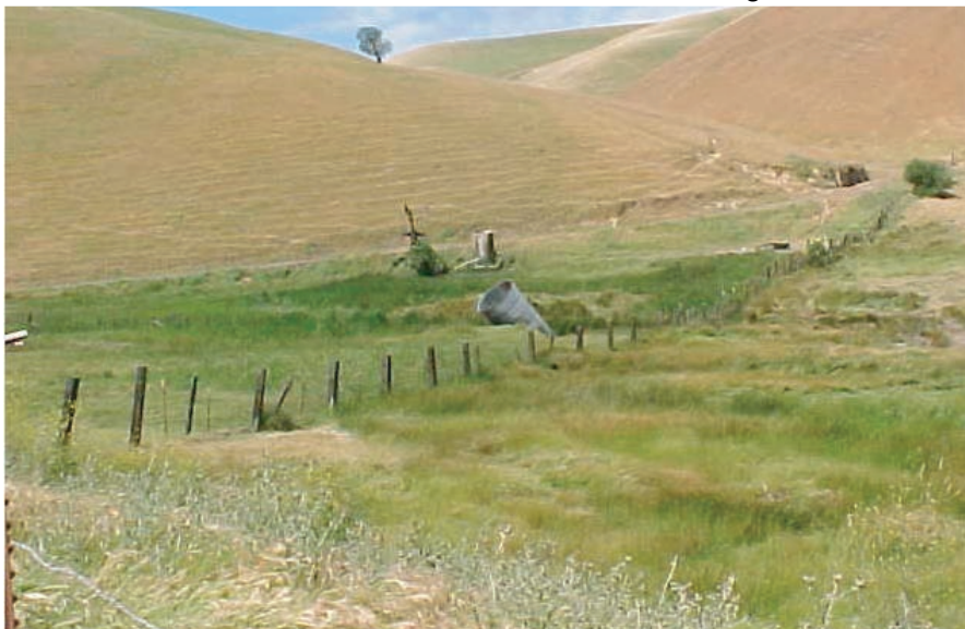
Seasonal PPEM wetland with a failed culvert
